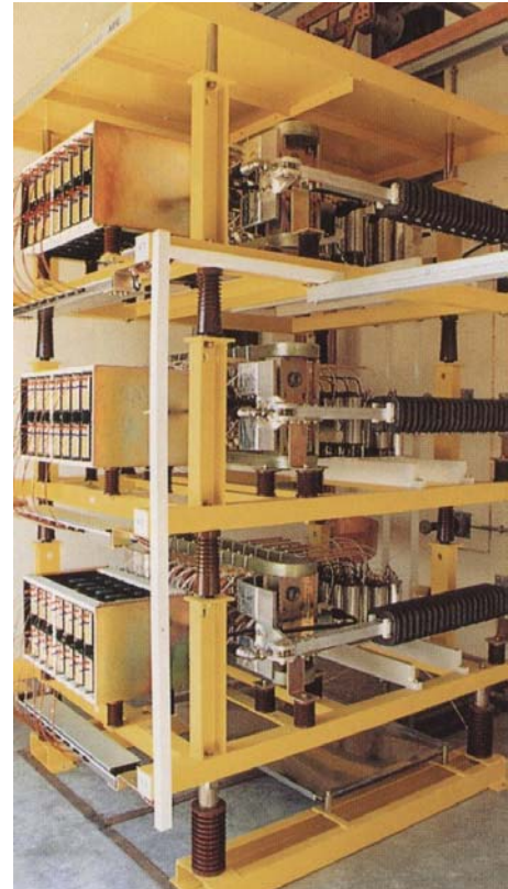
Adjustment and automatic control of electric currents are similar to pipe systems of liquid media for which valves are required. This picture shows a threephase thyristor valve (TCR valve) designed for power up to 60 MVA and is part of a power electronic system developed by AEG.
