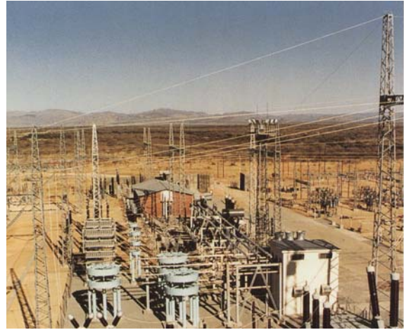
Transformer station Omburu with reactive power compensation plant from AEG. The installation reduces disturbances within the power supply grid and contributes to the fact, that voltage variations do not influence the power supply adversely.
