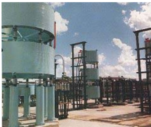
Fig 5 132 kV compensator plant
